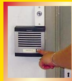
Door Entry System
